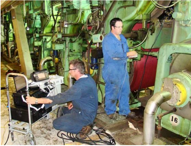
Figure 1: Ultrasonic examination of paper machine dryer cylinders to check for thickness variations, cracks and flaws
